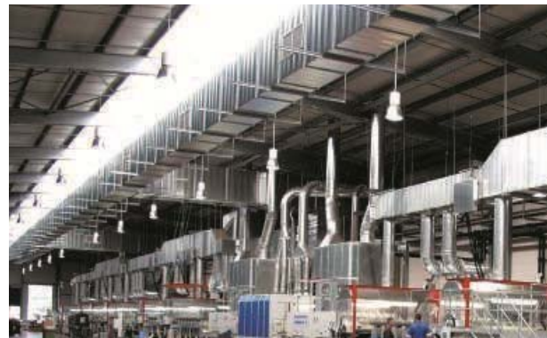
Figure 2: Factory Air Extraction for Mercury Vapour Lamp
